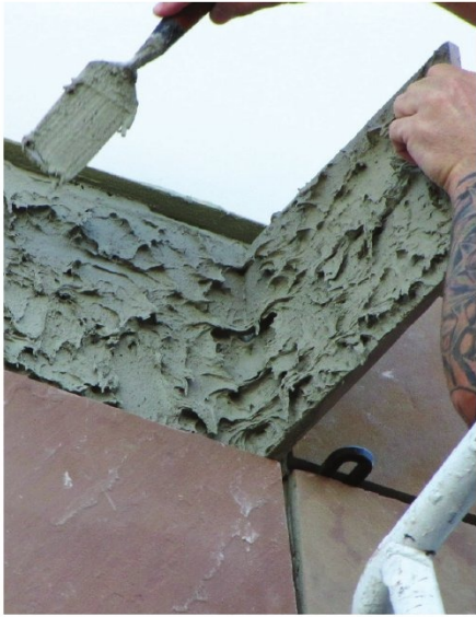
The quality control (QC) plan should verify relevant industry standards are being met, for example, achieving 95 percent thin-set contact between the tile and the substrate in a wet application.
