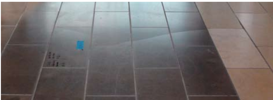
An indent fracture is caused by bottom of the stone shortening from deformation caused by the thin-set shrinkage, resulting in the crack. The top surface of the stone is drawn down at the crack location resulting in the indent.
