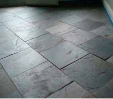
Natural stone slate floor installation that shows excessive tile lippage due to improper installation
