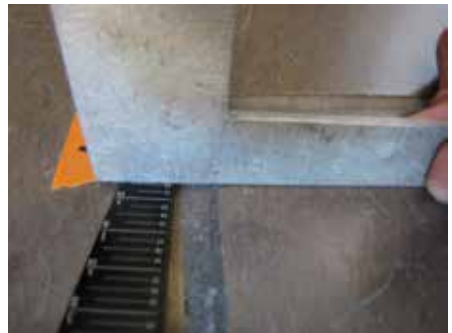
Measuring excessive tile lippage in stone at 4 mm (5/32") on a floor tile.
