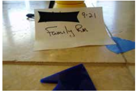
Limestone with excessive lippage.
