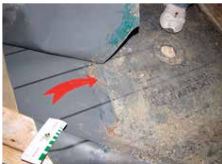
Seams, penetrations and transitions are the areas most vulnerable to problems, so special attention must be given to be sure they are sealed and flashed properly.
