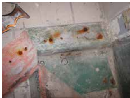
The waterproof membrane should never be penetrated, unless it is unavoidable, and then the penetration has to be properly flashed and sealed with the appropriate sealants to ensure it will never leak.
