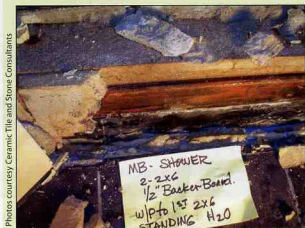
Moisture damage at a shower curb that had improper waterproofing.
