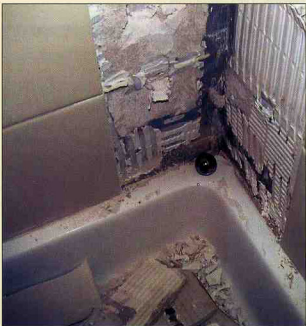
This shower had a prefabricated receptor using a backer board substrate. It lacked a transition joint, was not sloped to drain, and had inadequate adhesive coverage.
