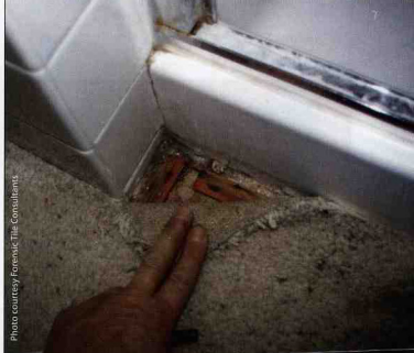
This photo illustrates carpeting at the shower receptor. There is water damage along the transition joint and under the carpet.
